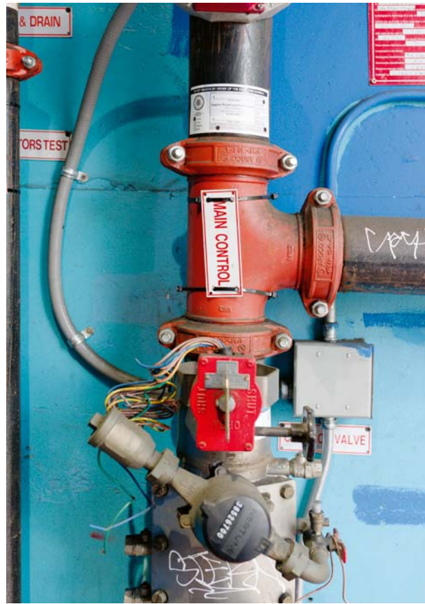
Control II | Kontrolle II
